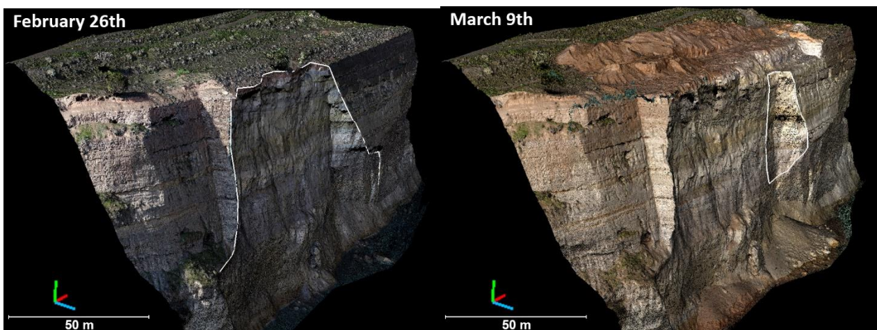
Figure 3. Point cloud of slope failure of Corinth Canal on February 26 th and March 9 th from Pix4D.
