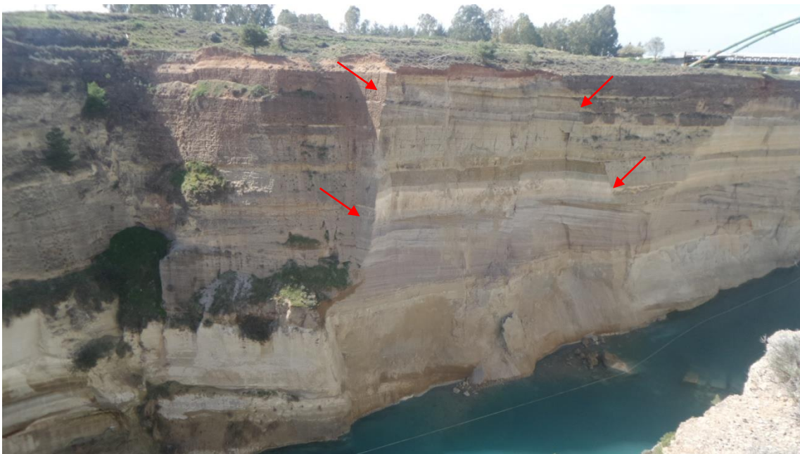
Figure 1. View of the slope failure, which occurred on February 26 2018 at the south slope of the Corinth Canal.
