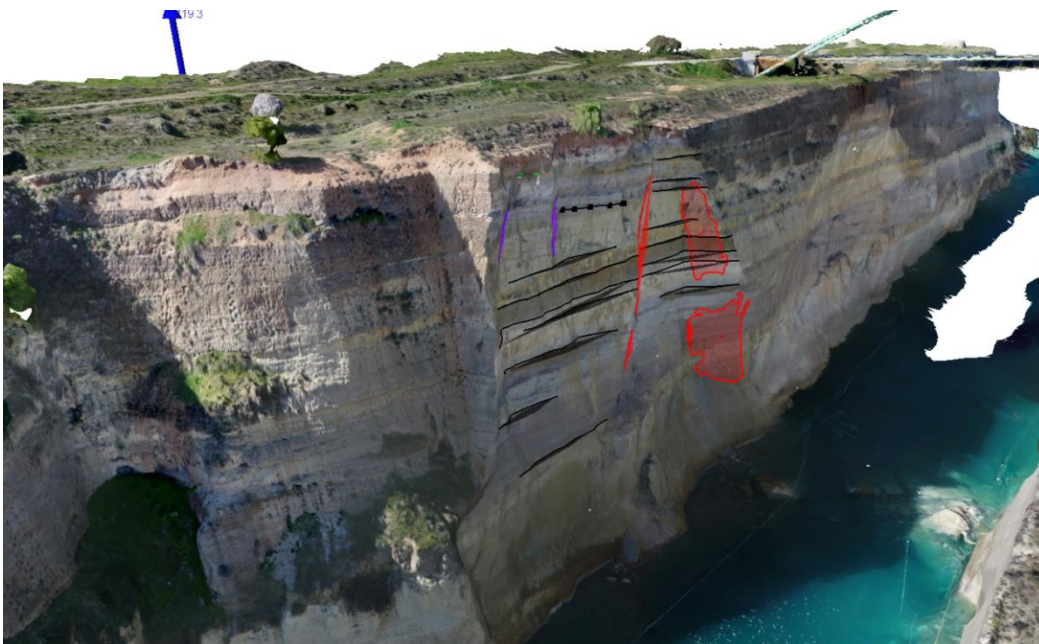
Figure 3. 3D Model from ShapeMetriX UAV illustrating faults and main discontinuity surfaces controlling the slope failure of 26 th February (fault surfaces in red, joint surfaces in blue, bedding surfaces in black).
