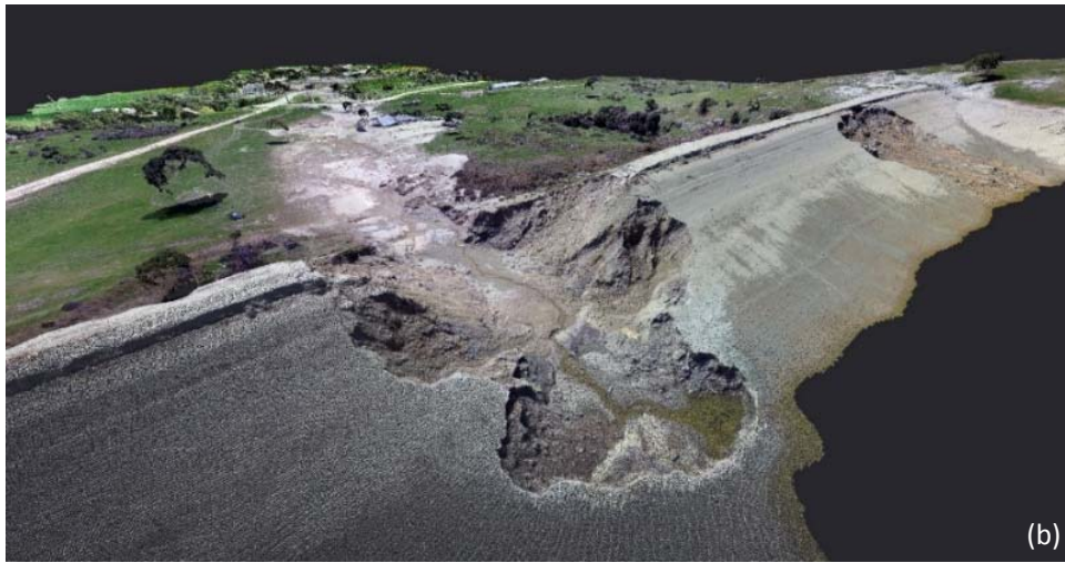
Figure 7. UAV-enabled 3D model of Sparmos Dam failure in Greece. (a) Orthophoto (plan view) illustrating also the disturbance in the downstream side of the dam (lower side in the picture); (b) 3D point cloud/model of the dam.
