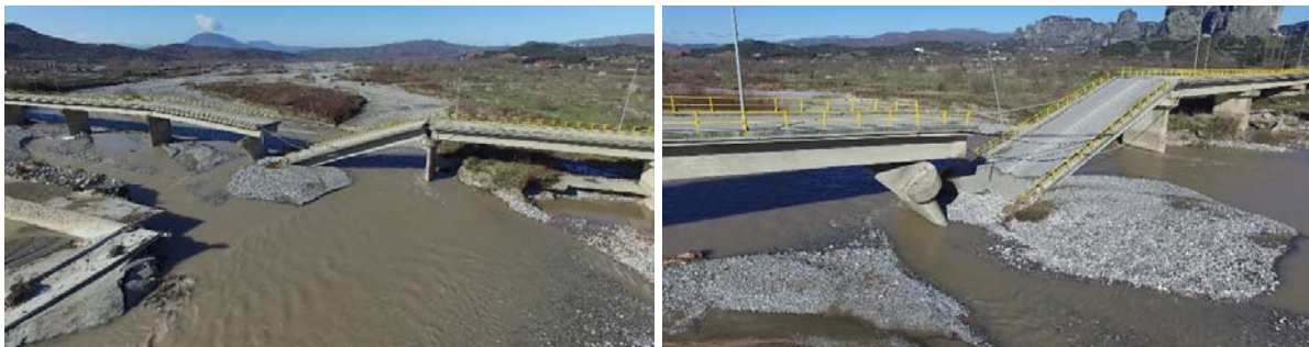
Figure 3. Oblique view of Diavas bridge from a distance and a closer view of the scoured bridge pier.
