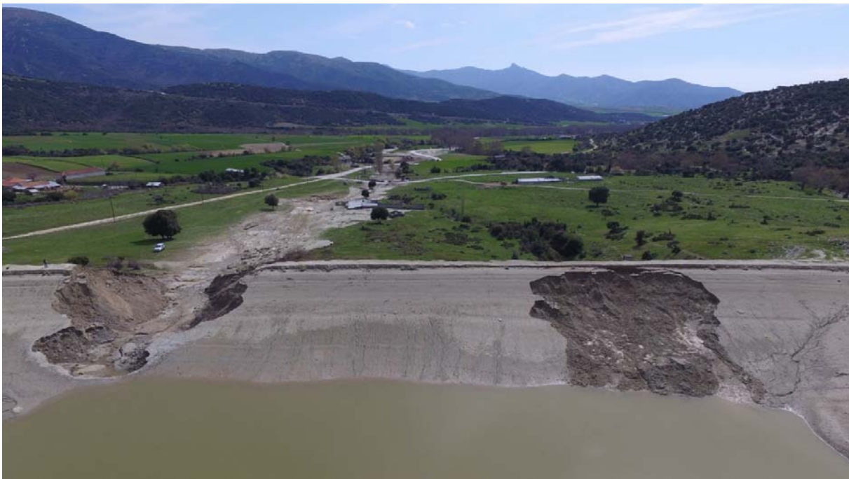
Figure 6. Aerial view of the Sparmos Dam failure.
