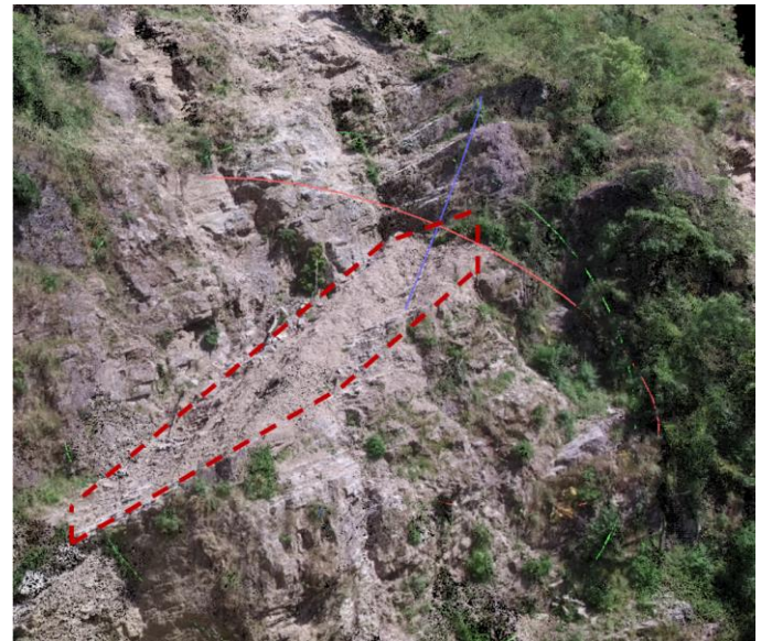
Fig. 11. Possible structurally-controlled failure in Landslide 2.
