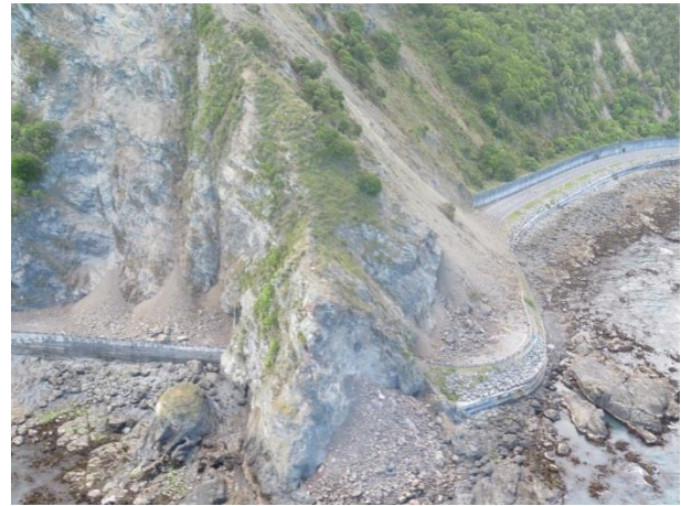
Figure 3: Landslides on either side of the Paratatahi Tunnels, State Highway 1, south of Kaikōura. The railway line at this location is enclosed in a rock shelter, and so was not directly affected. (Photo: S. Cox, 20/11/2016).
